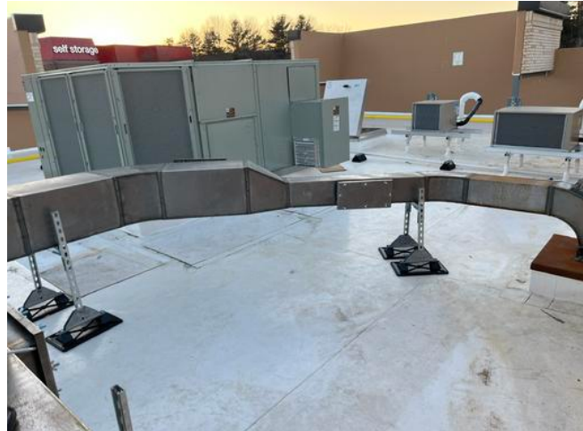
Grease Duct Supports
